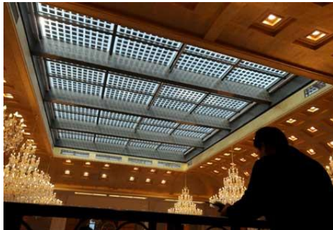
Image 5: Diangujinjiang International Hotel of Baoding, a 5-star hotel in China with solar panels installed (XinHua News, 2009)
